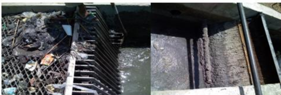
Primary screening unit
