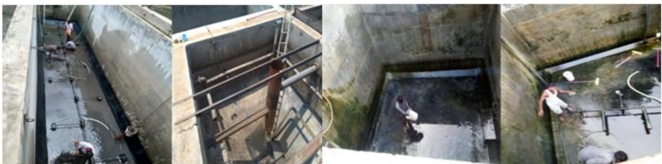
PRG STP CLEANING – Collection tank, settling tank, filtered water tank and reuse water storage tank
