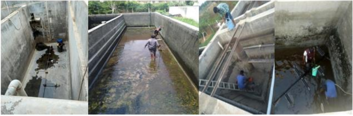
JMR STP cleaning – Collection tank, settling tank, filtered water tank and reuse water storage tank
