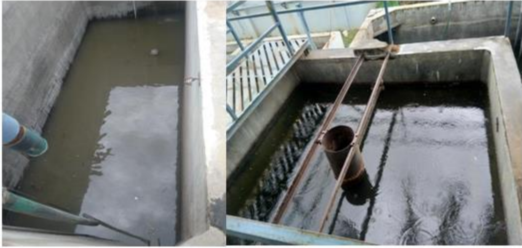
PRG collection tank, settling tank
