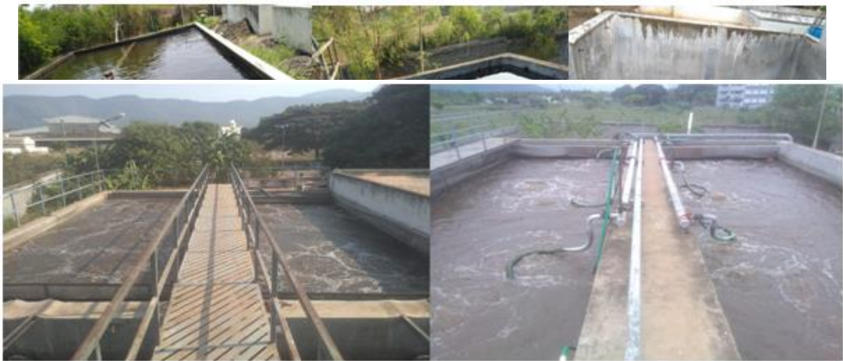
Storage tanks for treated water (before reuse in the garden)
