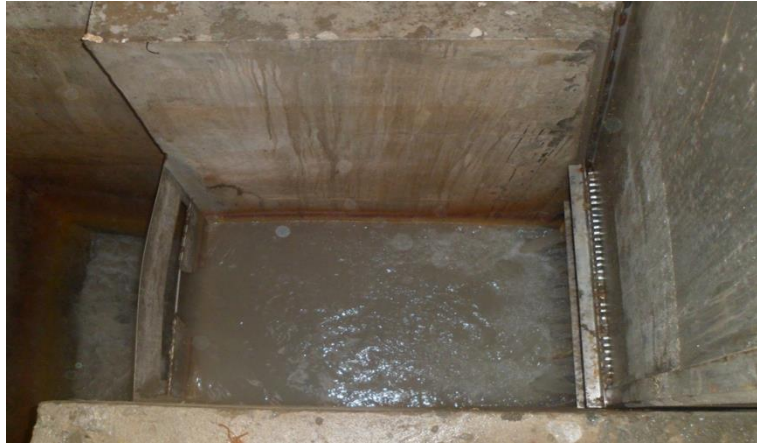
.Sludge drying bed
