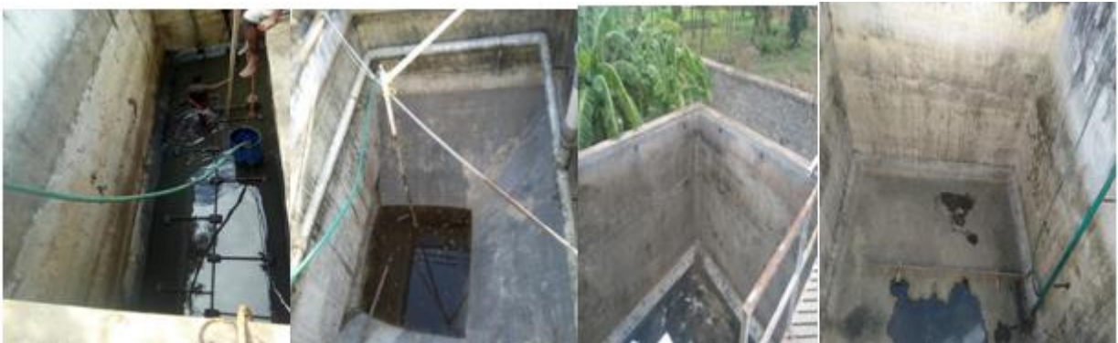
FDR STP Cleaning – Collection tank, settling tank, filtered water tank and reuse water storage tank
