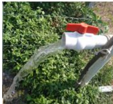
Outlet for the recycled wastewater from STP
